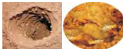
Termite & Termite mud galleries
